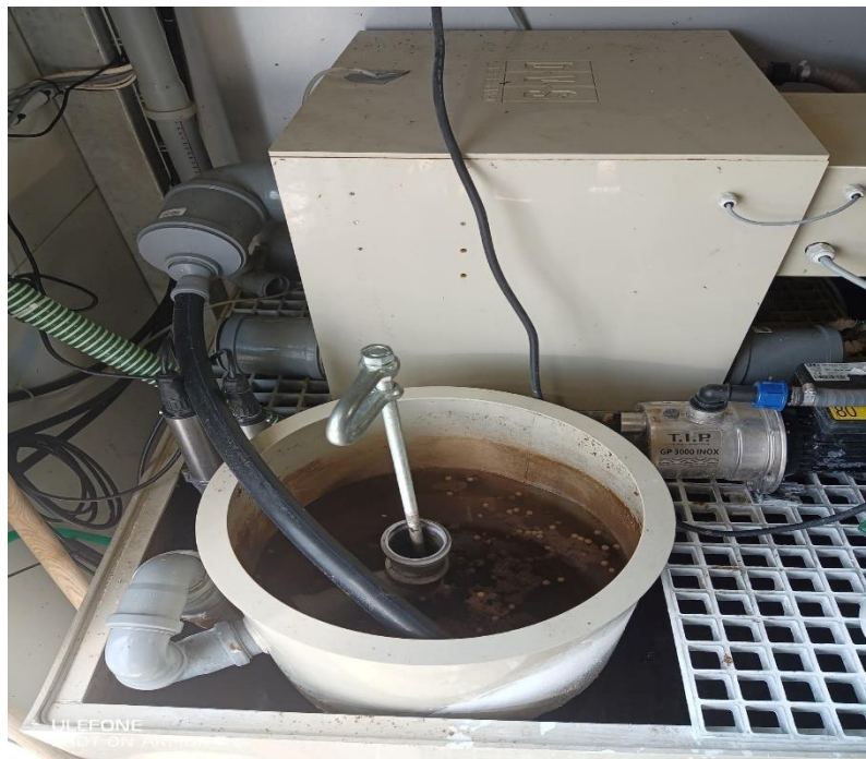
Figure 4. Mechanical filter and vortex where most of the waste is collected from the RAS (source: M. Prečanica).
