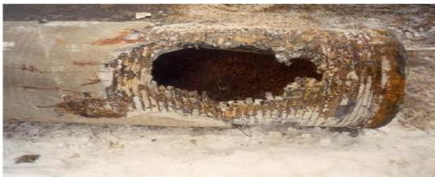
Slika 3-5. Korozije cjevovoda u tlu ( https://corrosion-doctors.org/SoilCorrosion/ , 14.08.2020.).
