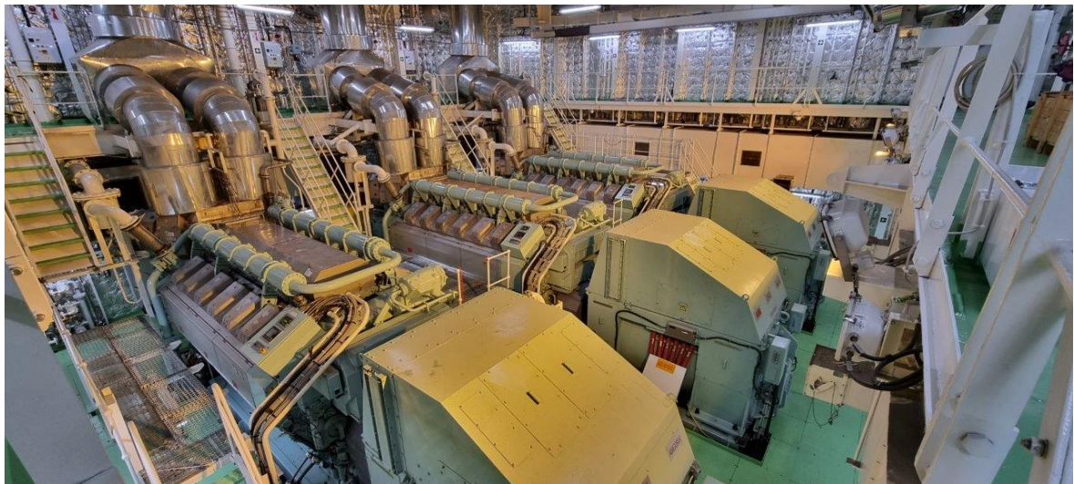
Figure 1-4 The three Wärtsilä 12V34DF gensets in the engine room of the LNG terminal (LNG Hrvatska, 2024)
